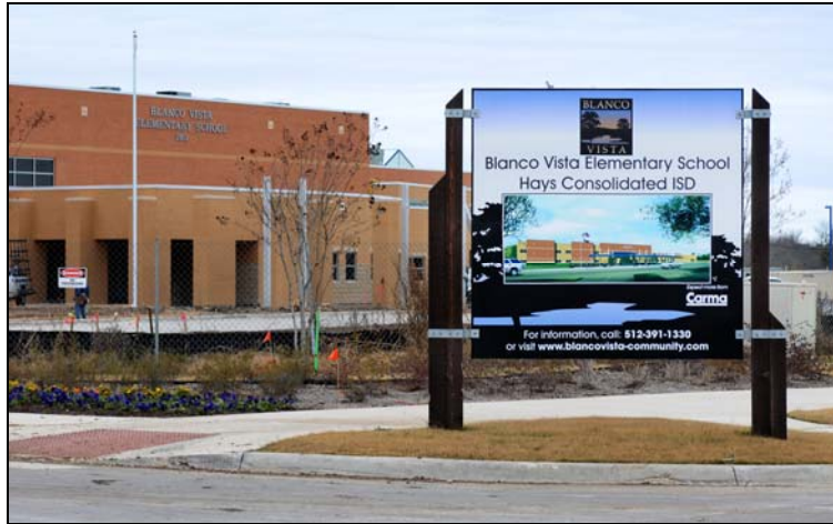
NEW SCHOOL for Hays CISD—Blanco Vista Elementary School under construction by the Hays District will open for students in fall 2008. (Photo by Don Anders)
